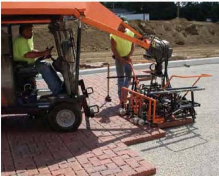
Figure 3. Mechanically placed pavers enabled an average installation rate of about 4,000 sf (400 m 2 ) per day including layout, screeding, mechanical laying, cutting edge pavers, joint-filling, compaction and clean-up.
