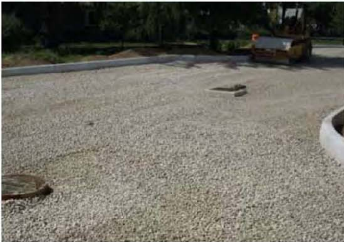
Figure 1. The No. 57 stone base is in place and being compacted with a vibratory roller. The No. 57 stone was placed over a No. 2 stone subbase.
